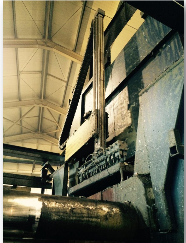
AUTOMATIC SPRAYING UNIT
